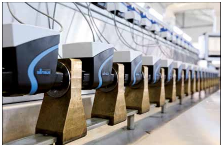
Fig. 4 Installed Sensus system
